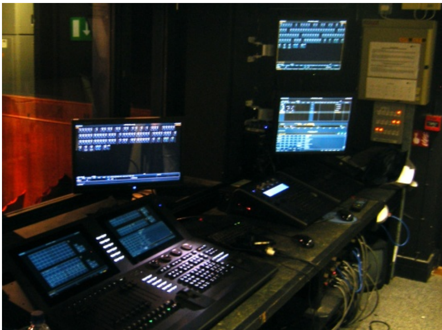
The lighting board
